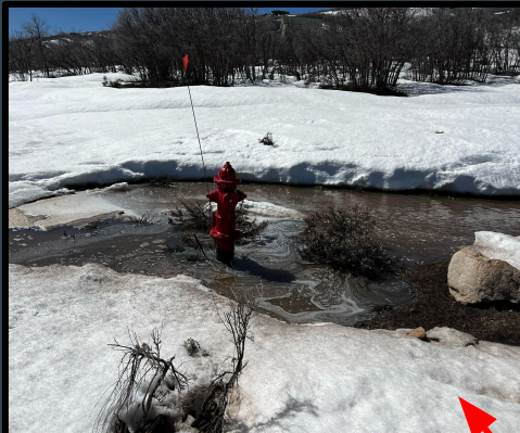
A clogged culvert
