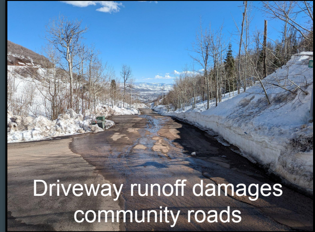
floods and erodes our roads
